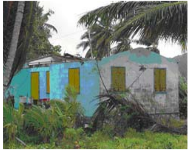
Photo 5: Damage to housing infrastructure
