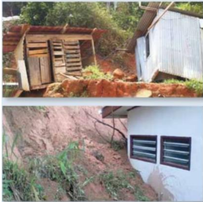
Source: Seychelles Government, Seychelles Damage, Loss and Needs Assessment 2013 Floods
